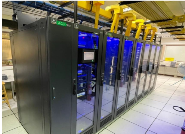
▲ Closed typed facility-cold/hot channels separation
